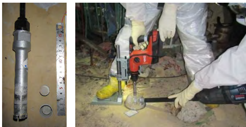
Figure 15. Sampling tool designed for remote operation (left) and a scene of concrete sampling in the Unit 4 reactor building (southwest corridor on 2F) (right)
